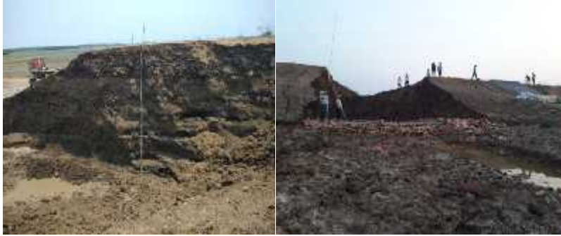
Fig.2. Photos showing breached sections of summer storage (SS) tank
